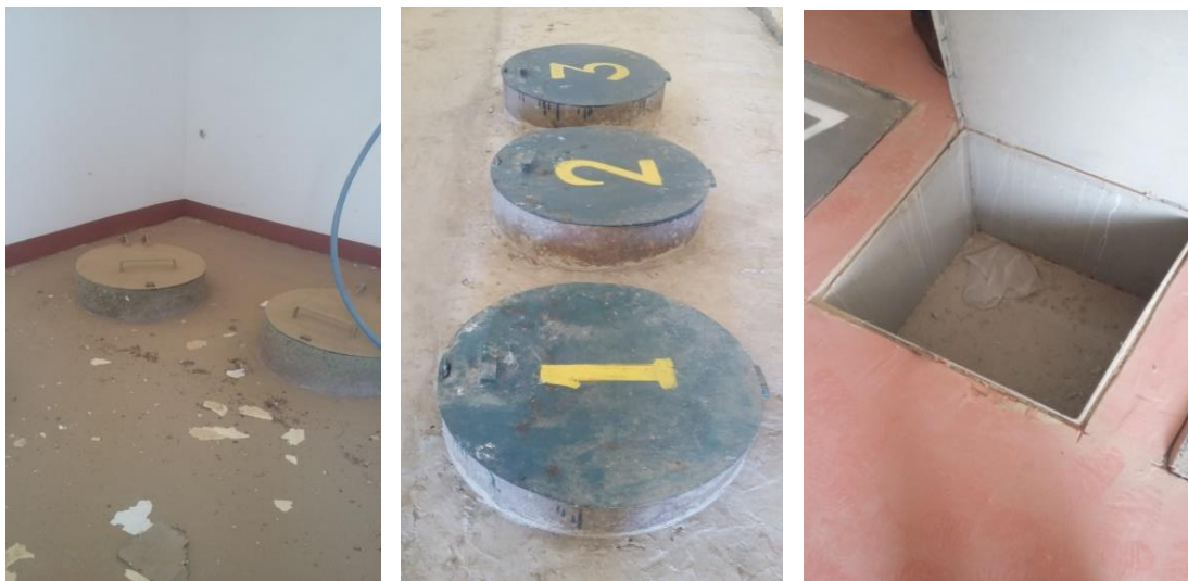
Fig.(26): Internal shape and setup of the temporary storages.
