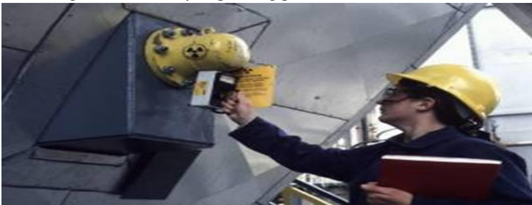
Fig.(28): Typical level gauge for detecting fluid high and low levels
